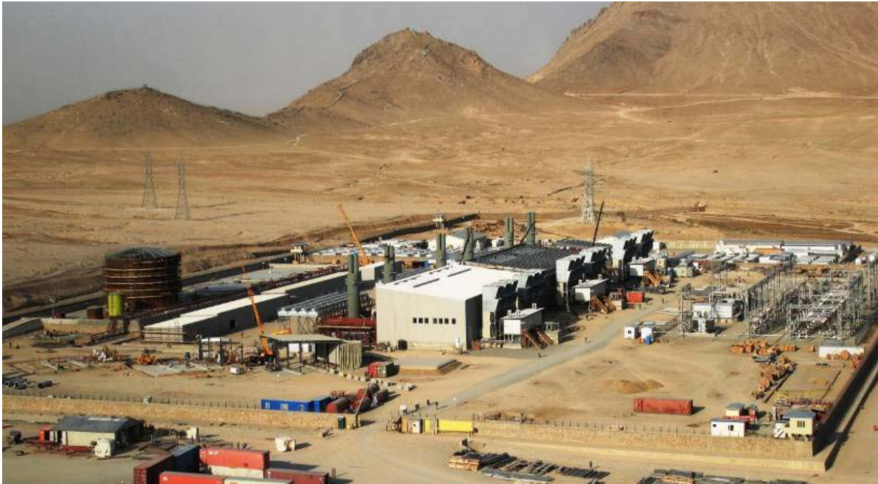
Photo of Kabul Power Plant as of October 21, 2009
