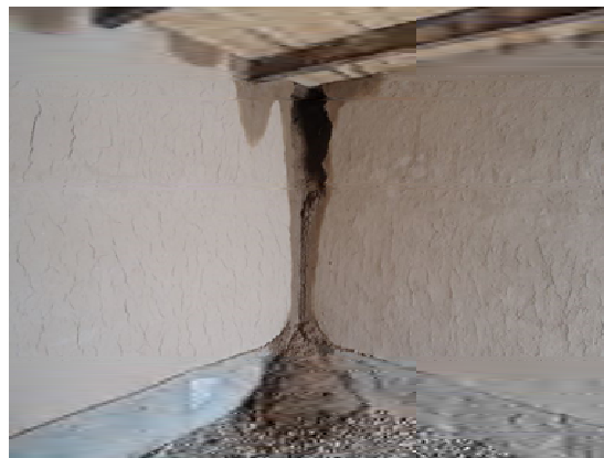
Photo 3 - Interior View of Building Deterioration Due to Water Penetration
