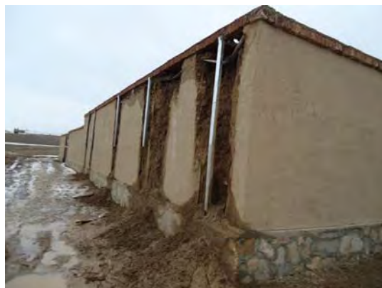
Photo 2 - Exterior View of Building Deterioration Due to Water Penetration
