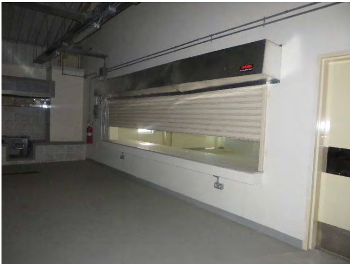
Photo 2 - Non-certified and Non-fire-rated Rolling Counter Door in the DFAC
