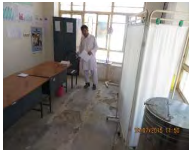
Photo 2 - Treatment Room at Facility 2933
