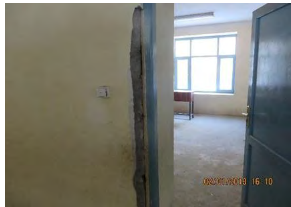
Photo 15 - Interior Crack at 8 Classroom Takhar School
