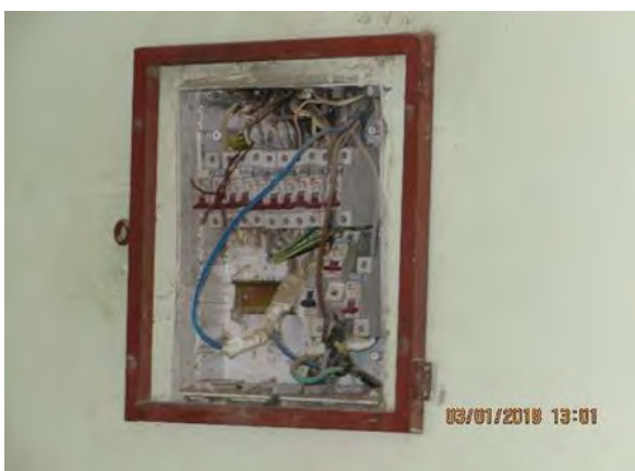
Photo 1 - Exposed Wiring in Hostel Building
