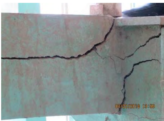
Photo 5 - Cracks in Hostel Building I
