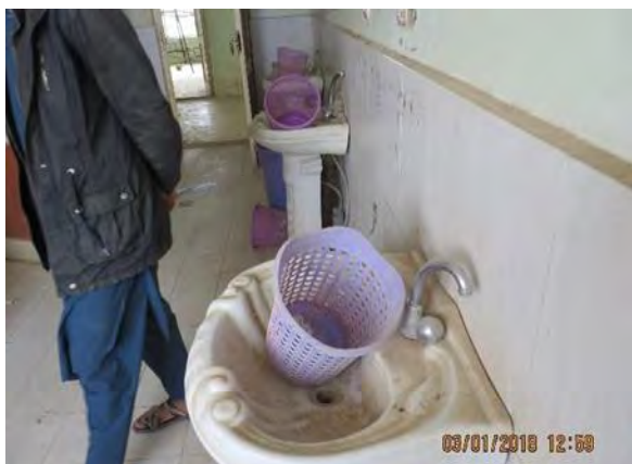
Photo 3 - Unsanitary Sinks in Hostel Bathroom
