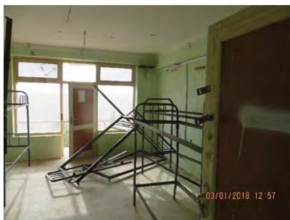
Photo 2 - Broken Bedframes in Hostel Room
