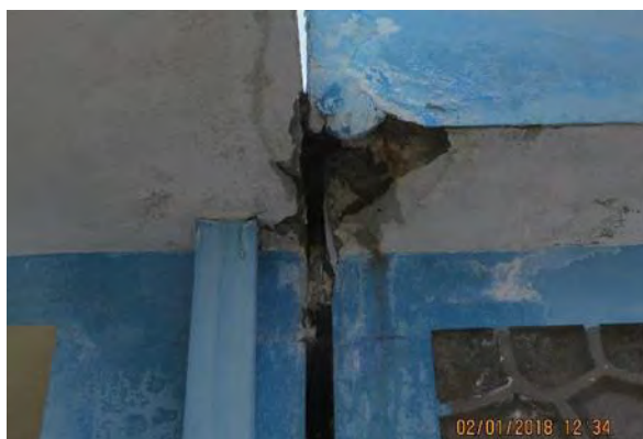
Photo 13 - Exterior Crack at 8 Classroom Takhar School
