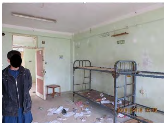
Photo 4 - Trash and Unsanitary Conditions in Hostel Room
