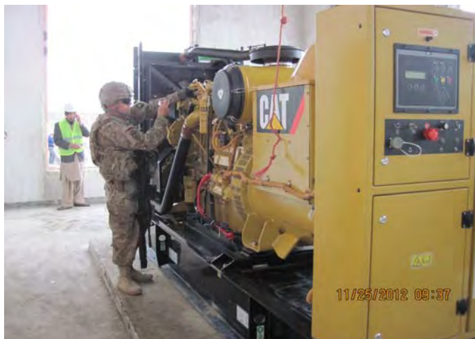
Photo 1 - Generator Installed for Gardez Provincial Hospital
