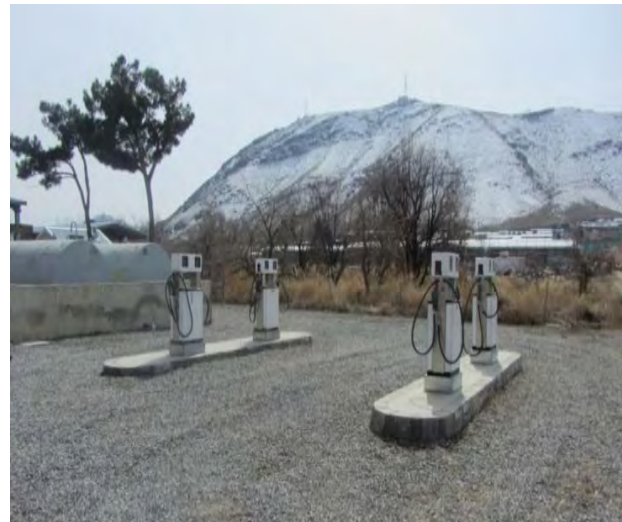
Photo 2 - Fuel Point with Tanks and Pumps
