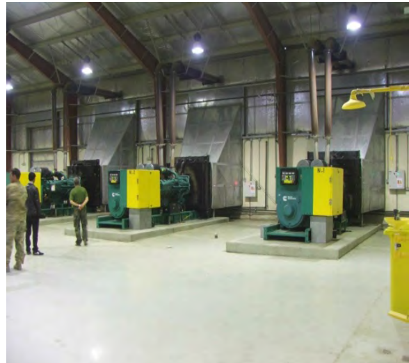
Photo 1 - Power Plant with Generators
