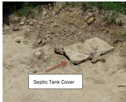
Photo 2- Lid Covering a Gravity Absorption Septic Tank
