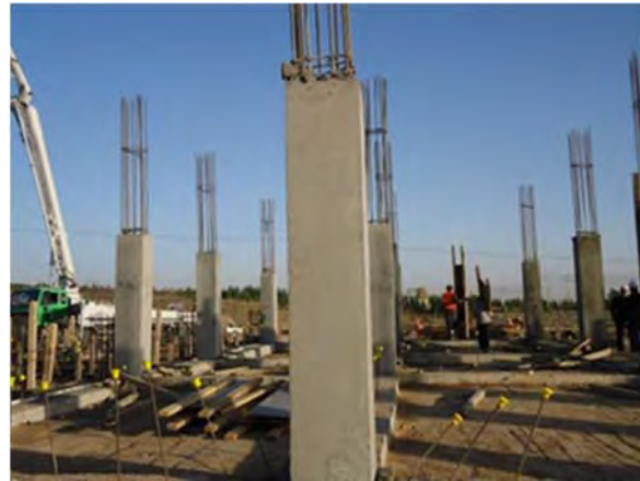
Source: U.S. Army Corps of Engineers, December 11, 2013
