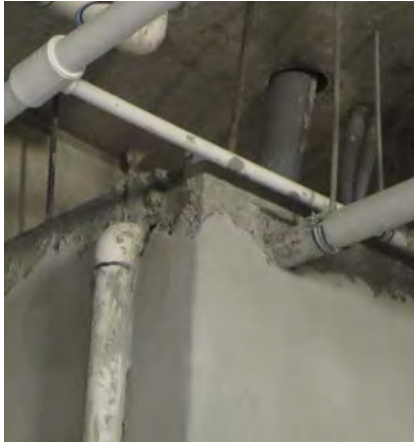
Photo 4 - Pipes in the Dormitory's Second-Floor Shower Area Installed through Partition Wall without Pipe Sleeves
