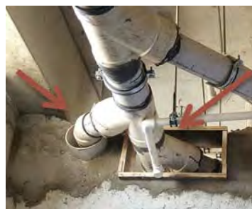
Photo 3 - Sewage Pipes in the Laundry Area Installed through Partition Wall with Proper Pipe Sleeves
