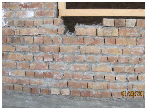
Photo 3 - School Building's Exterior Brick Wall with Gaps in the Mortar
