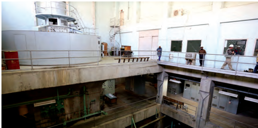
The turbine hall at the Kajaki hydroelectric station in Helmand Province currently has two turbines like the one visible at left. U.S. aid will provide for installation of a much-needed third turbine delivered in 2008. (State Department photo)
