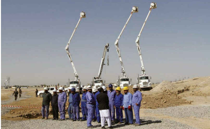
USAID broke ground on its 10 MW solar power plant project in Kandahar on September 24, 2017. (USAID photo)
