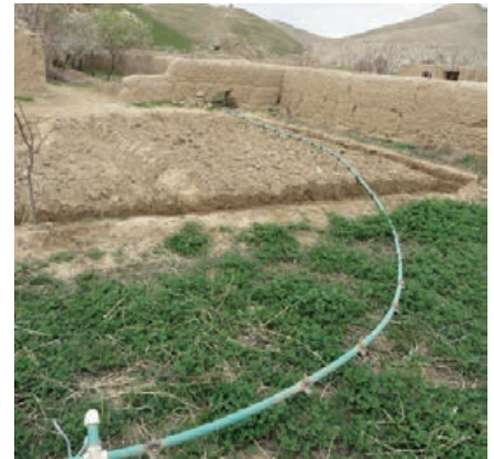
Strengthening Watershed and Irrigation Management (SWIM) -supported irrigation piping in Qezel Kend District, Balkh Province. (SIGAR photo)
