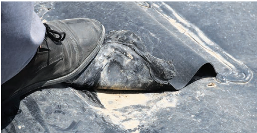
Detached pond liner air vent at wastewater treatment facility. (SIGAR photo)
