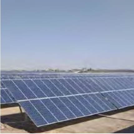
The USAID-supported 10 MW solar power plant in Kandahar Province. (USAID photo)
