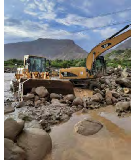
Construction crews work to clear the Parwan-Bamyan road after August flooding. (Taliban regime photo)
