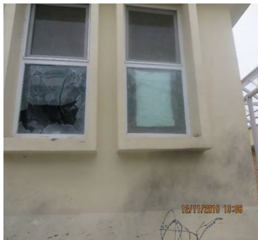
Photo 1 - Broken Window at Health Facility 1167
