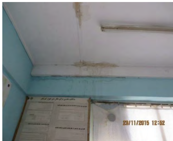
Photo 2 - Possible Leaking Roof at Health Facility 1982
