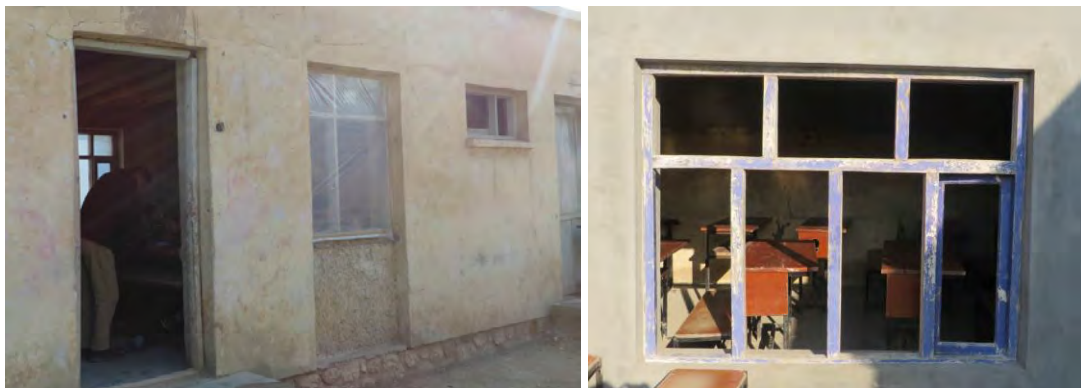
Photo 10 – Missing Windows and Doors in Classroom at School S043 Ain Balkh District
