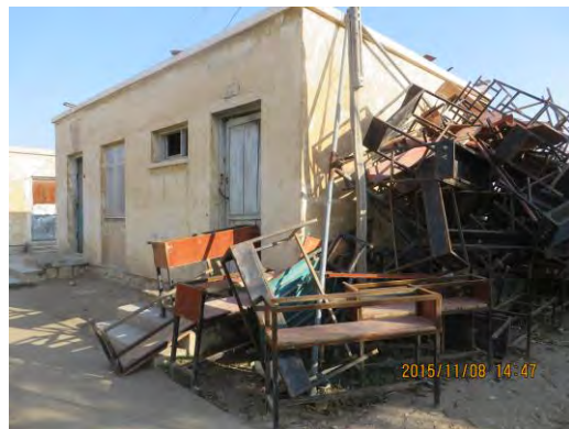
Photo 12 – Stockpile of Broken Furniture Outside School S038A
