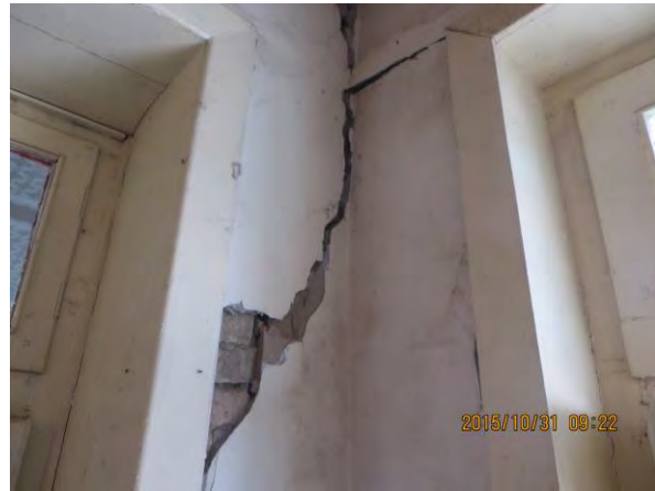
Photo 9 – Structural Damage on the Interior Wall of School SR11
