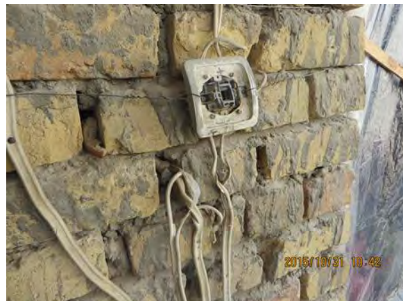
Photo 4 – Damaged Electrical Sockets at School SR10 in Mazar-e-sharif District
