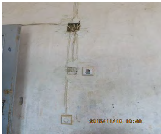
Photo 3 – Exposed Wires from Electrical Socket at School SR07 in Khulm District
