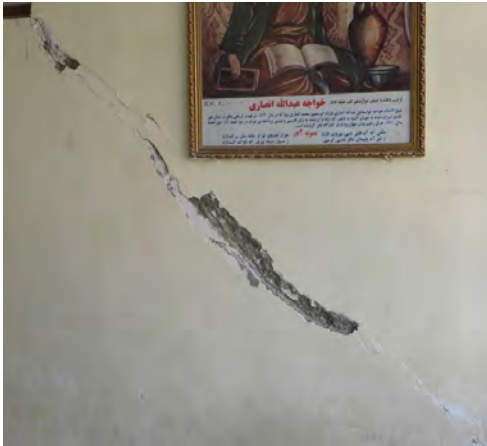
Photo 8 – Structural Damage on the Interior Wall of School S039A
