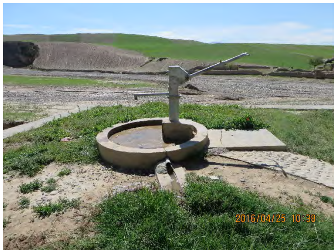
Photo 6 - Functioning hand pump at facility 1617 in Takhar
