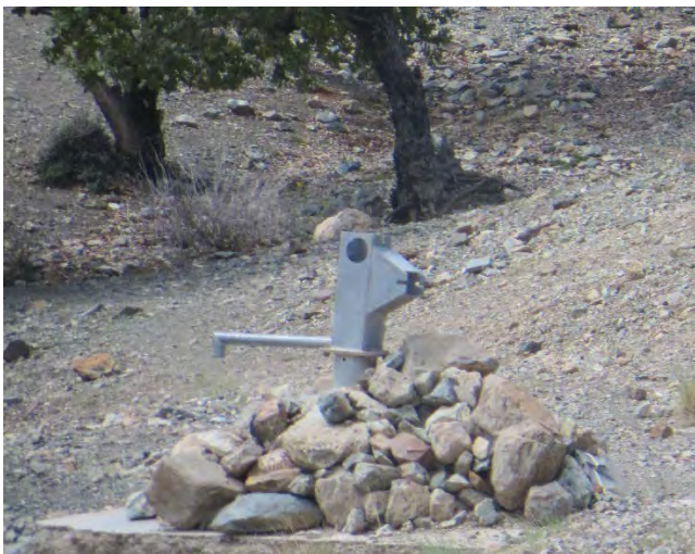
Photo 5 - Missing hand pump at facility 2131 in Khost
